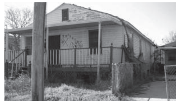
The marks of the original search parties are still visible on this house still standing nearly two and a half years after Katrina hit.
